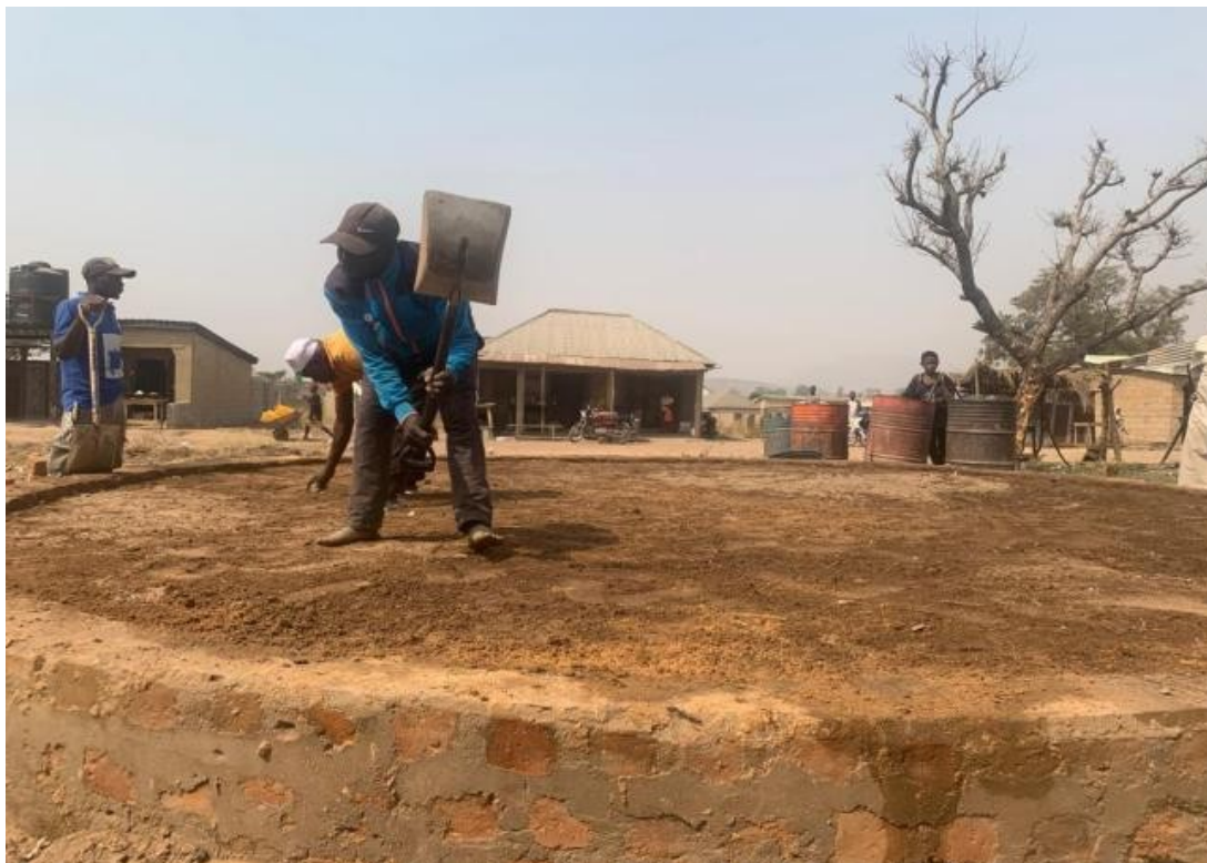
Community members flatten the foundation for a new Hello Hub in Dakwa. Photo courtesy of Hello World and CITAD.
